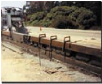
The first contractor used concrete mix that was too wet and the barrier crumbled. The second contractor had to redo some of this work.
